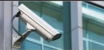
CCTV Camera System
